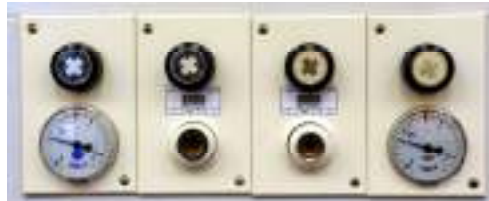
Fig. 16-1 Central oxygen distribution panel
