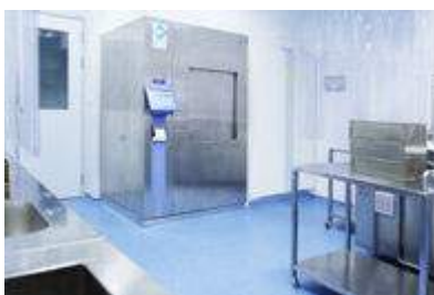
Fig. 2.4-1 Automatic disinfection and washing machine, separators
