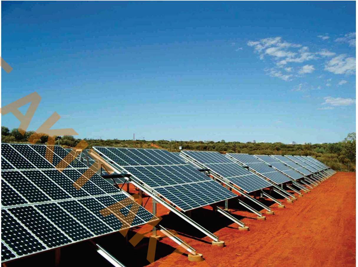
Fig. 3.1: An array of solar panels
